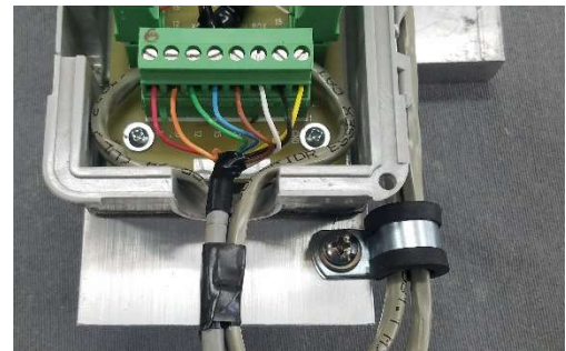
FIGURE 112 Controller plug inserted into header, using cable management.
